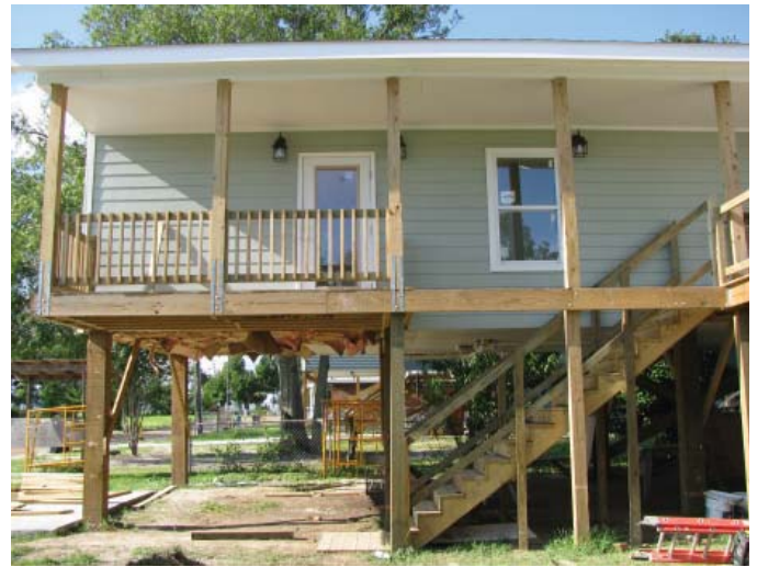
(FIG.A) DRIVEN WOOD PILES are a quick and straightforward foundation system, but must be installed professionally.
