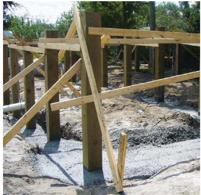
(Fig.5) The wood piers are placed on site and connected with a concrete grade beam. Once the concrete is set, the bracing can be taken away and work on the floor framing can begin.
