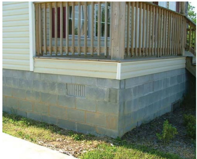
(Fig.12) Stem walls in flood zones have special venting requirements. Consult local code officials for specifics.
