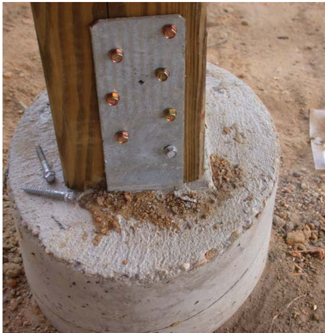
(Fig.16) Connections between concrete piers and wood posts should be placed accurately for ease of framing.
