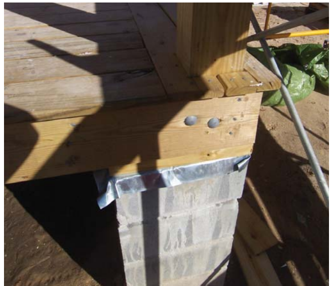
(Fig.10) The steel connection from the rim joist to the top of the CMU pier should be accurately placed for ease of framing.
