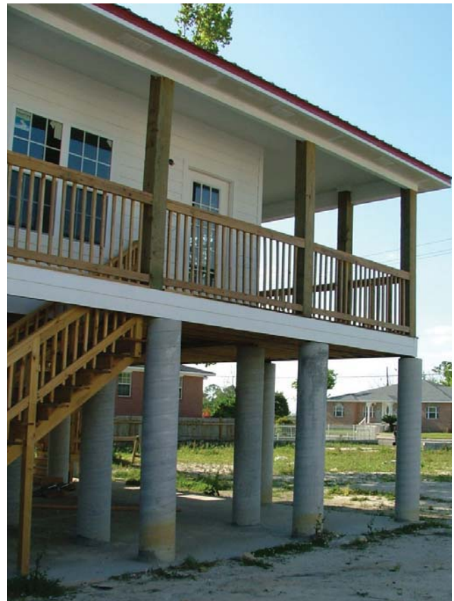
(Fig.13) Poured concrete piers can be cast in many forms, and at many heights, making this a very versatile foundation choice for storm and flood zones.
