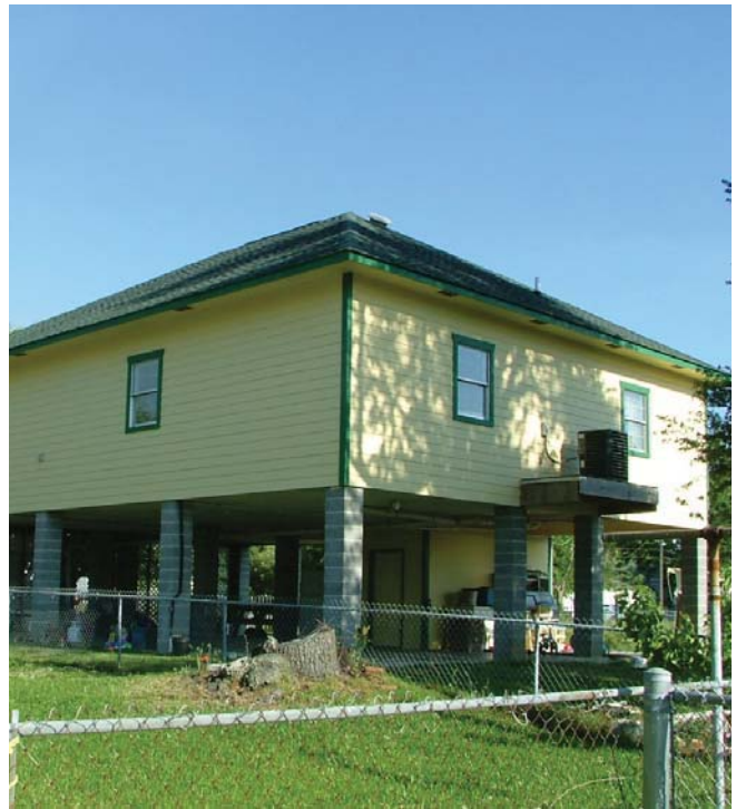
(Fig.9) Elevating houses a full story on CMU piers is discouraged due to susceptibility to lateral wind forces.
