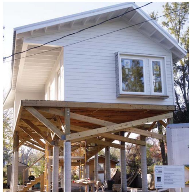
(Fig.15) Concrete can also be poured part way to the finished floor, with bolted wood posts making up the remaining distance.
