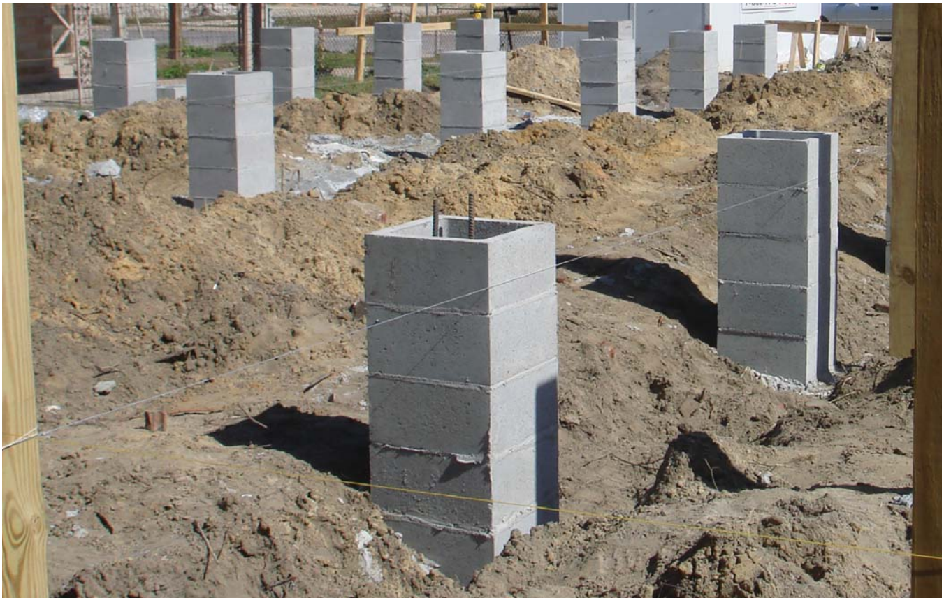
(Fig.8) The CMU piers should be laid by experienced masons to ensure the foundation is square and can resist lateral wind forces.
