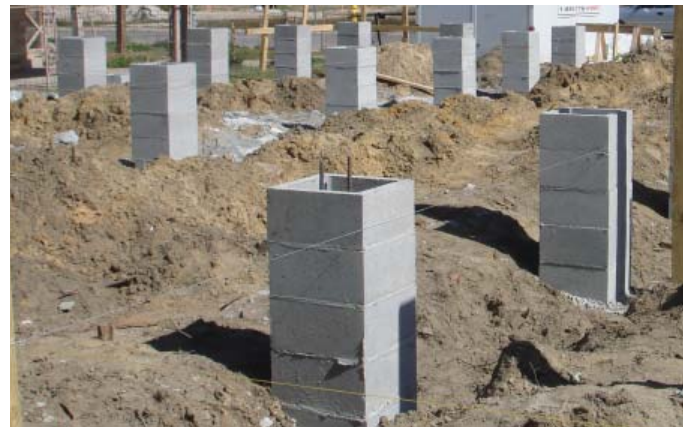
(FIG.B) CMU PIERS bear on a continuous footing and are grouted with rebar to resist uplift forces.
