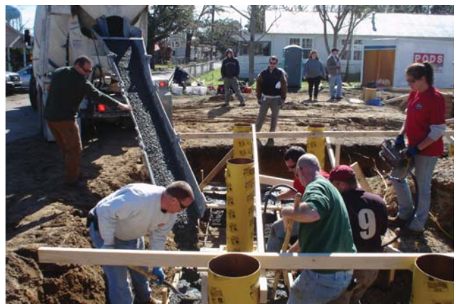
(Fig.18) Round cardboard tubes are a common, simple, and fast formwork for piers.
