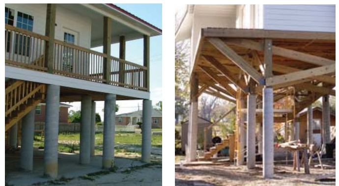
(FIG.C) POURED CONCRETE PIERS can either extend to the floor system rim joist (left), or connect to intermediate wood piers (right).
