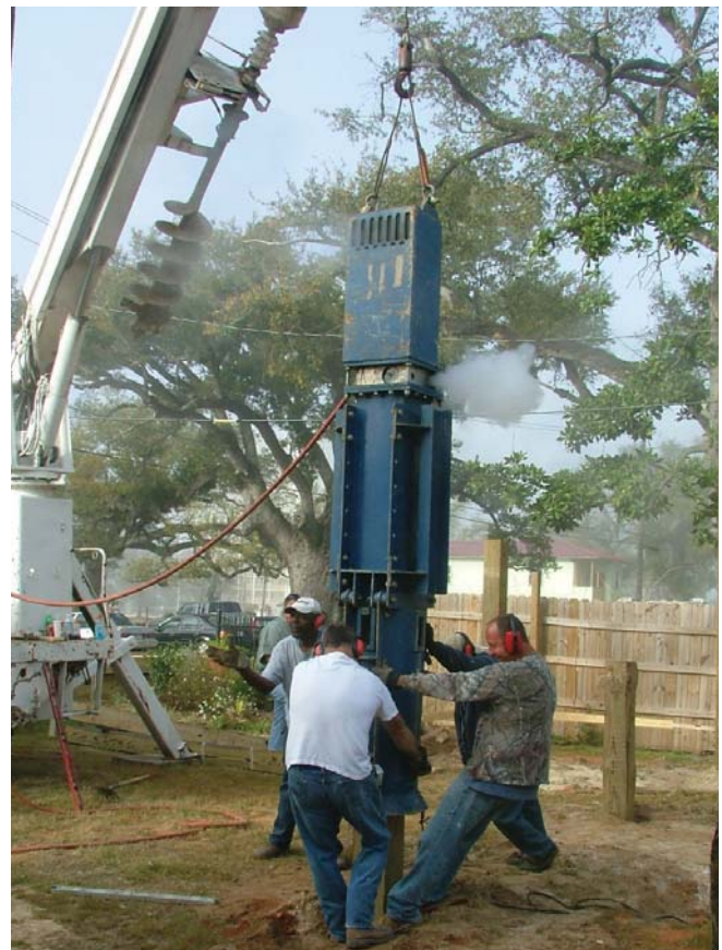
(Fig. 2) Professionals keep the timber in place while the pile-driving hammer drives it down.
